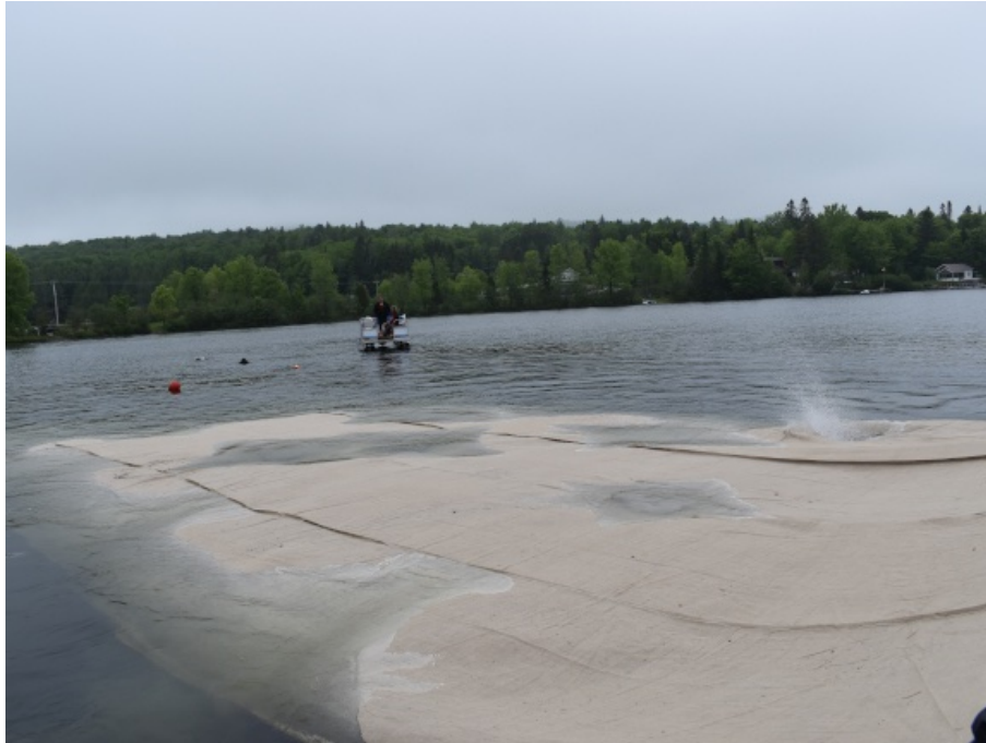
Figure12 : Installation of jute tarps at Lake Sergent. Photo credit: Stéphane Pelletier (Pelletier, 2021).
